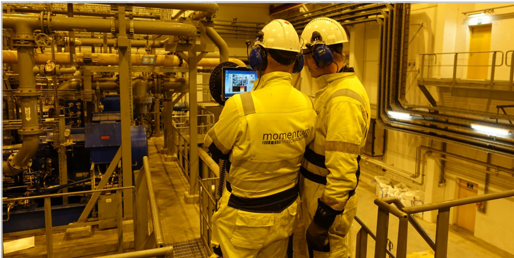
Leakage detection. (Photo: Momentum Technologies AS)
